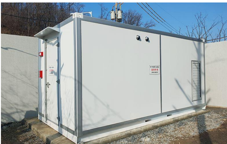
2024 Seoul City Building ESS (for peak reduction) - Yangjae AI Support Center (300kWh)
