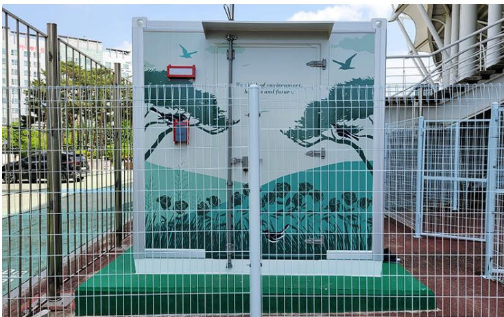
ESS for buildings in Goyang City in 2023 (peak reduction) - Goyang Sports Complex (200kWh)
