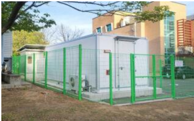
2021 ESS for building in Incheon (peak reduction) - National Institute of Environmental Research (1000kWh)
