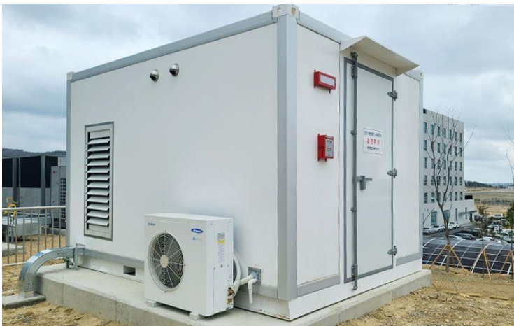
2024 Pohang City Building ESS (for peak reduction) - Gyeongsangbuk-do Eastern Office Building (160kWh)
