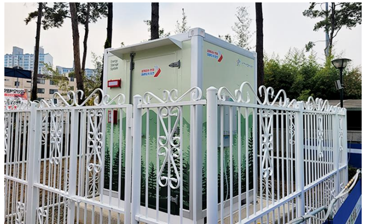
ESS for buildings in Osan City in 2023 (for peak reduction) - Osan Sports Center (100kWh)
