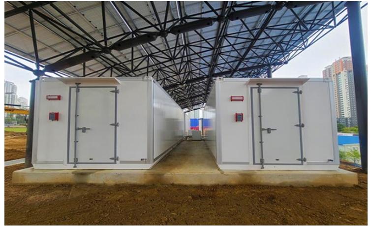
ESS for building in Gyeonggi-do in 2021 (for peak reduction) - Gyeonggi-do new office building (1992.54kWh)
