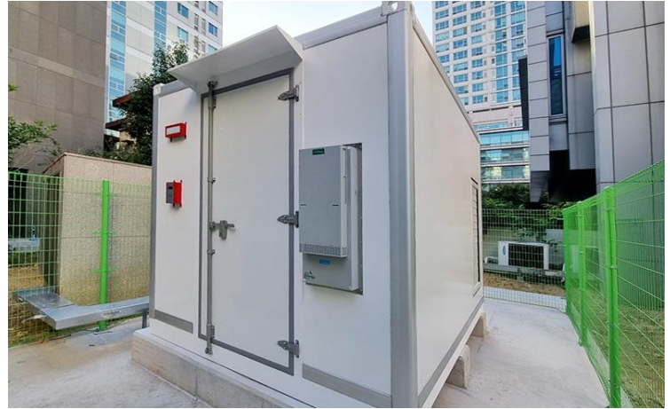
ESS for buildings in Busan city in 2023 (for peak reduction) - National Pension Service Busan Regional Headquarters (200kWh)
