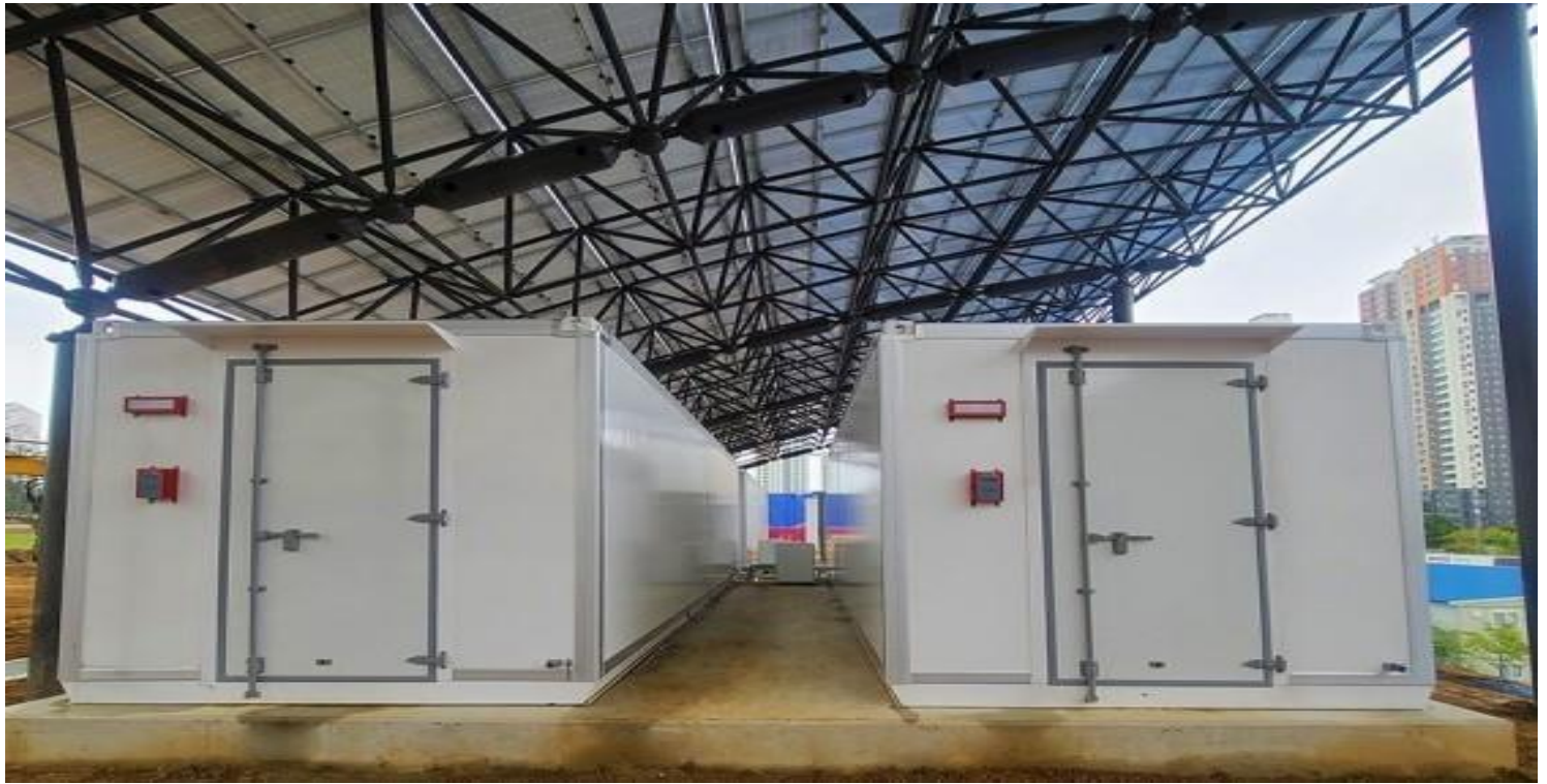
▶ Gyeonggi-do City hall(1.9MWh)
