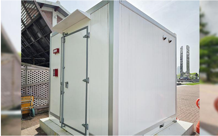
2024 Jeonju City Building ESS (for peak reduction) - Hwasan Gymnasium (300kWh)
