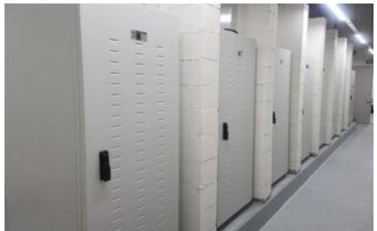
2021 ESS for building in Bundang, (peak reduction) - Bundang Combined Cycle Power Plant (320kWh)
