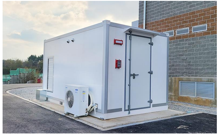
ESS for buildings in Wanju-gun in 2023 (for peak reduction) - High-risk plant disease and pest isolation research and testing building (200kWh)
