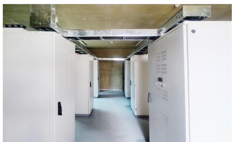
2021Y Hongseong Building ESS (peak reduction) - Hongseong Automotive Certification Center (200kWh)
